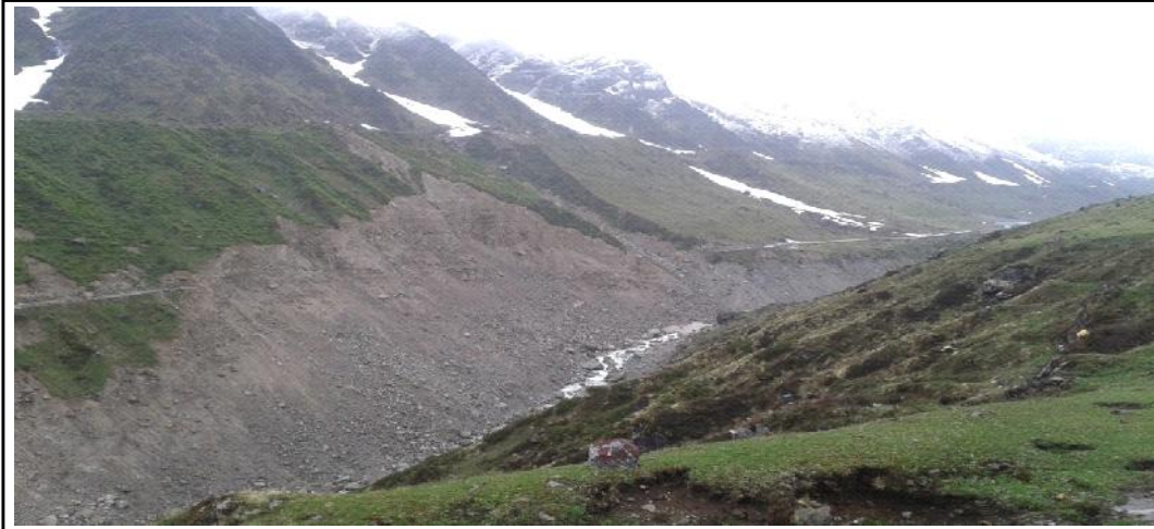
Photo taken by researcher (Road damaged due to flash flood at Kedarnath)
